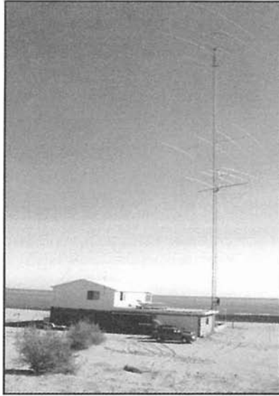
Photo 5: A populated guyed tower at the former XE2DV on the eastern shore of the Sea of Cortez. W7ZR was the owner.
