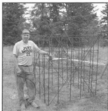
Photo 3: The finished cage after a couple of hours. Note the X bracing on each face. The extra lengths will be cut off with a hand grinder.
