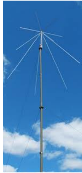
Wideband HF vertical antenna mounted on a guyed pipe mast.
