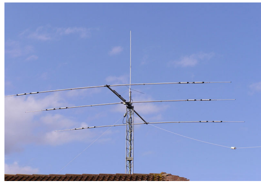
Rotatable HF Yagi beam with VHF vertical above and a wire dipole attached to the free-standing metal-lattice mast.
