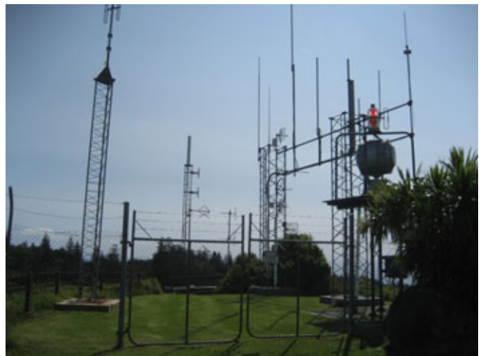
FM Broadcast and Comms tx site, Mt. Pitt, Norfolk Island
