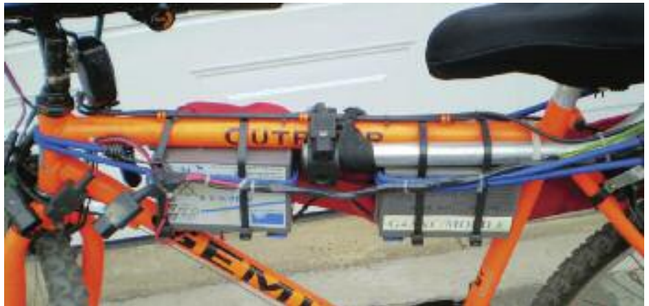
PHOTO 4: The primary pair of 7AH batteries that provide power to the radio.
